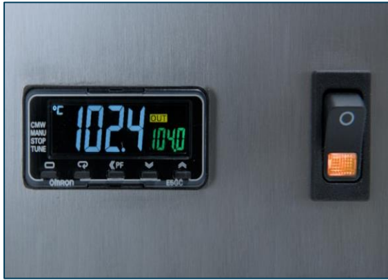
Control panel with digital display
